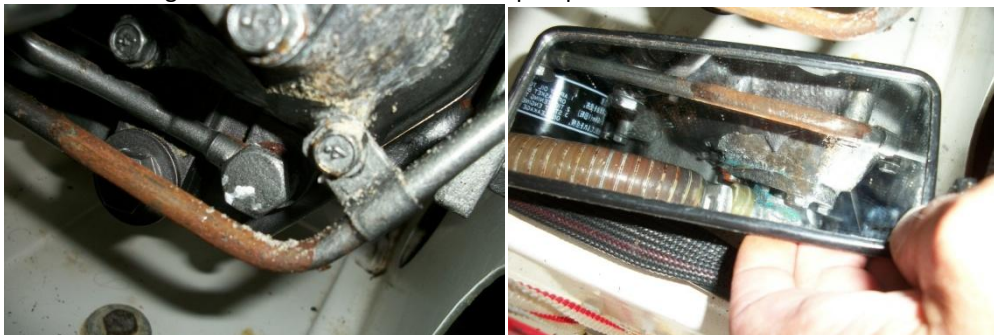
Fig 9 -10 Corrosion on oil pipe and cleaned underside.
