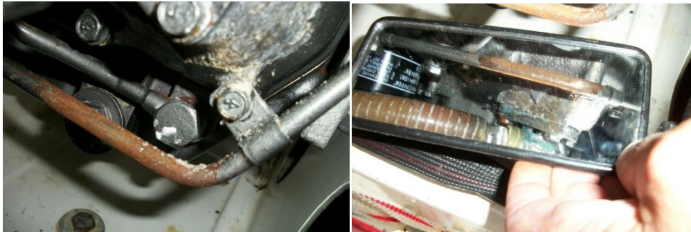
Fig 9 -10 Corrosion on oil pipe and cleaned underside.
