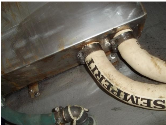
Holding tank stains
