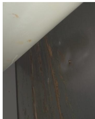
Stains from top of tank
