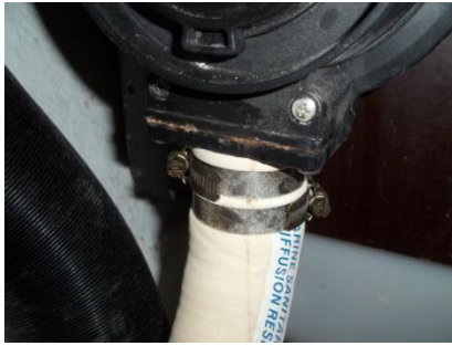
Minor leak at holding tank pump.
