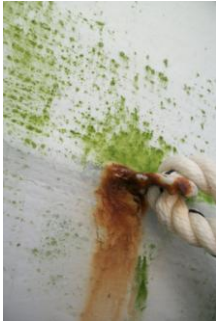
Fig 1 Corroded bitter end
