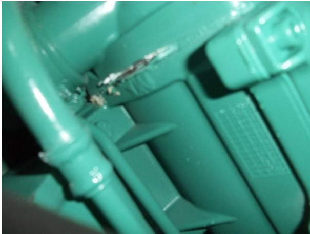
Leak under intercooler gasket
