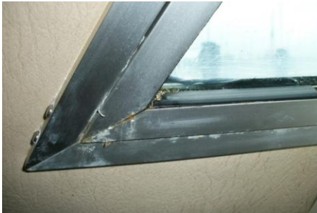
Fig 18 leak port cabin window, starboard same.
