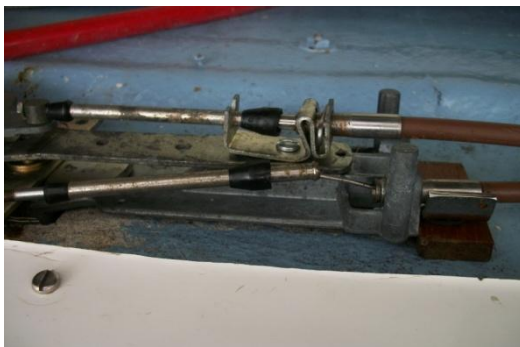
Fig 24 TX control not protected and cable broken.
