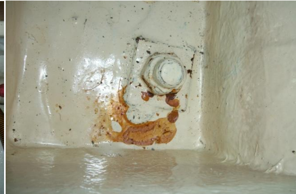
Fig 2 Keel stud and corrosion stain
