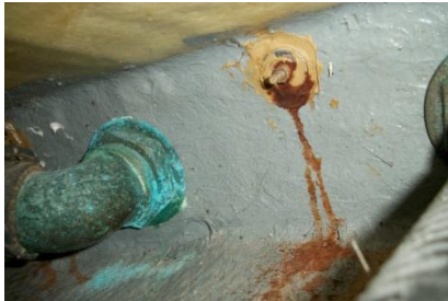
Fig 22 Mild steel rust.
