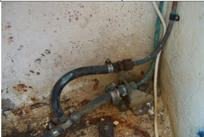
Fig 11 gas locker fittings corroded.
